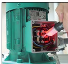
Incorrect phase sequence
